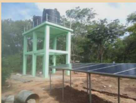
Water towers and solar panels ©GNAP
