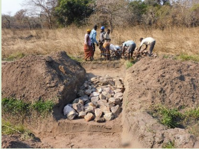
Road drainage system ©GNAP
